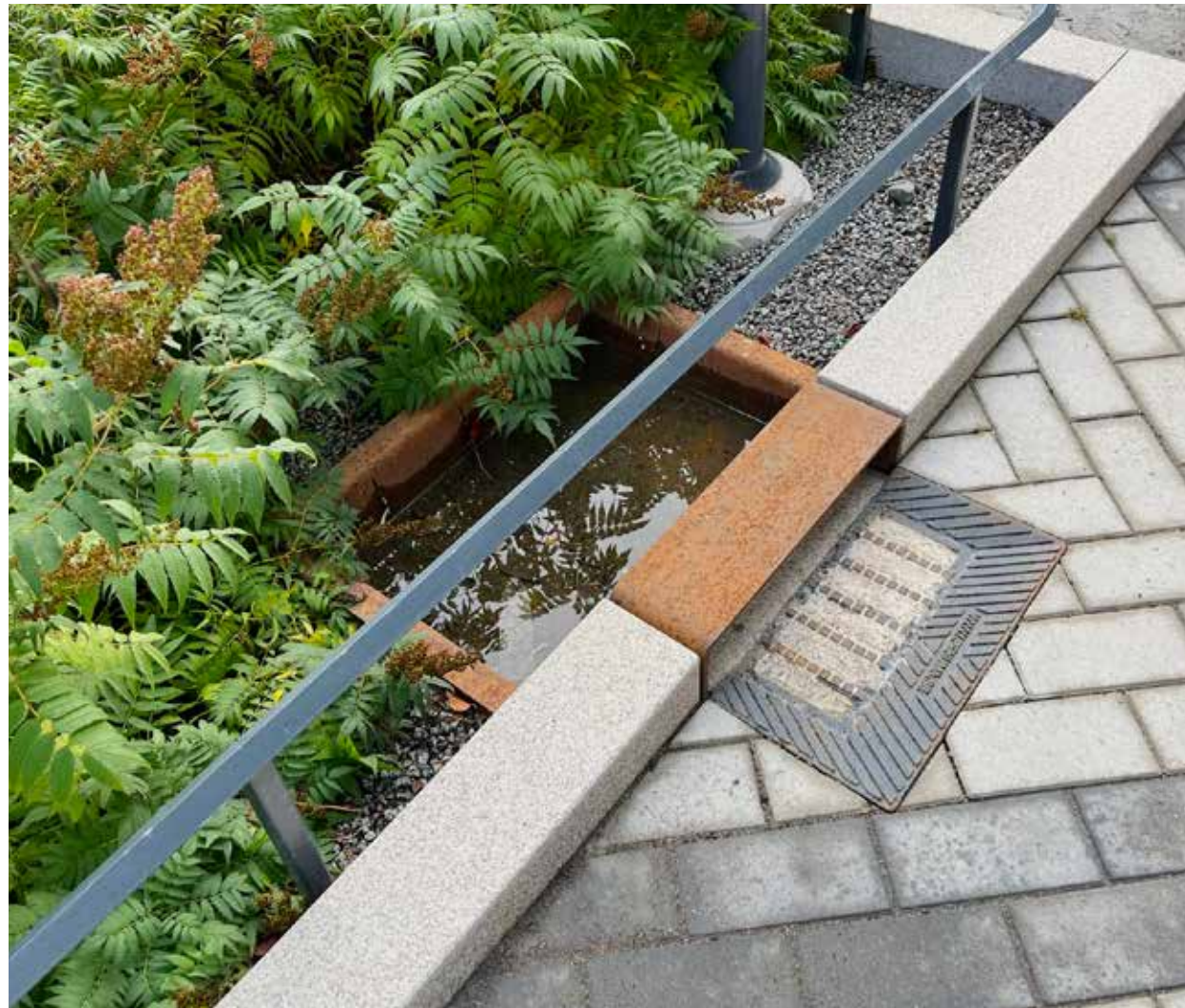
Sand / silt trap at raingarden inlet
