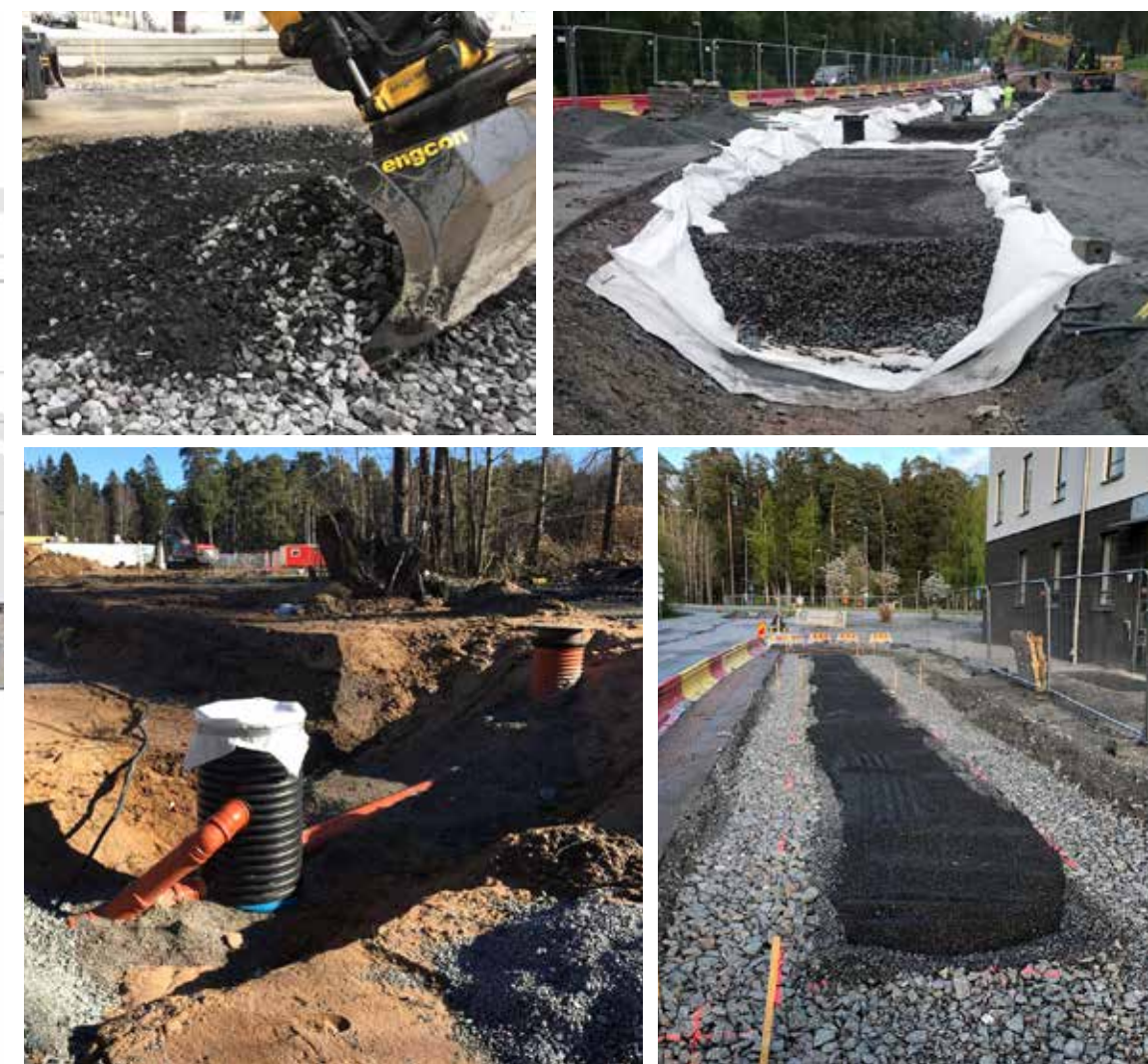
Control well with overflow
